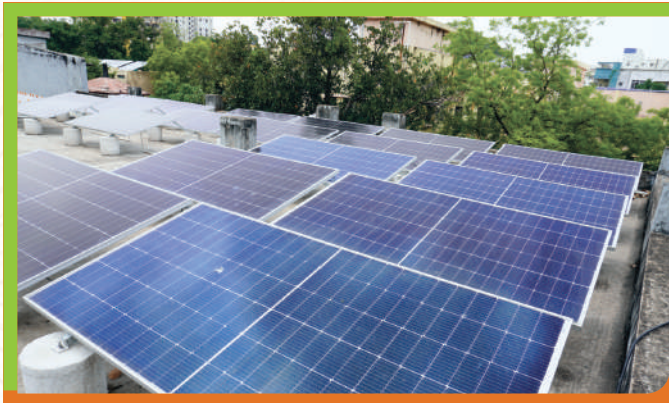
Grid Tied Solar System 96.93KVA
