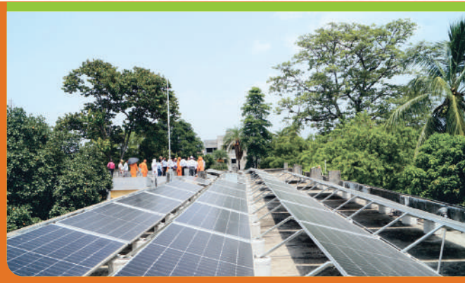
Grid Tied Solar System 96.93KVA
