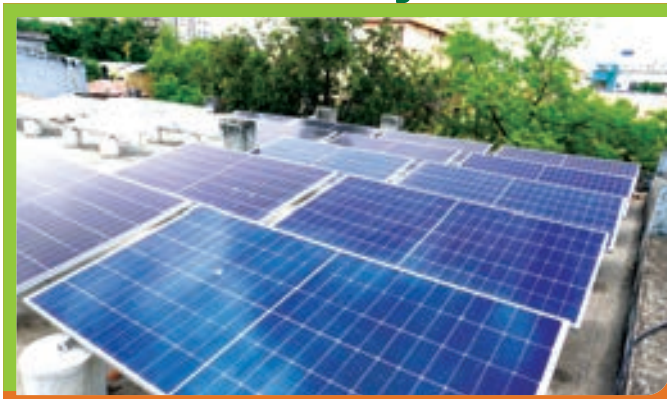
Grid Tied Solar System 96.93KVA
