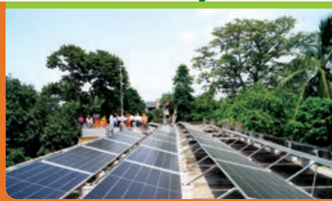
Grid Tied Solar System 96.93KVA
